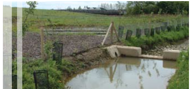
Weir inlet into a reedbed and three GCN breeding ponds – construction and monitoring
